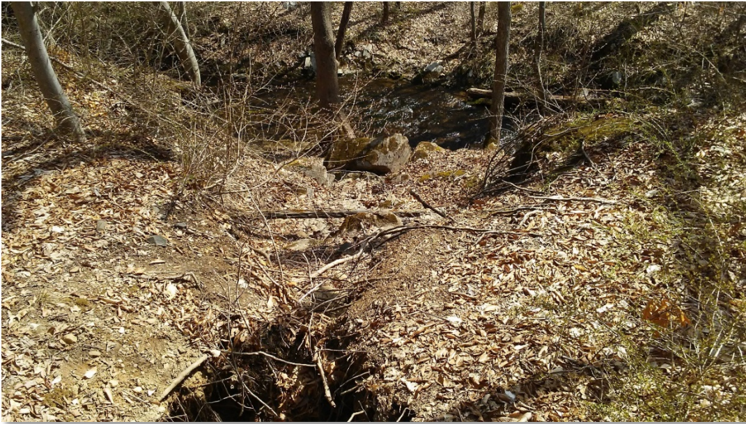
The channel to the brook is somewhat eroded.
